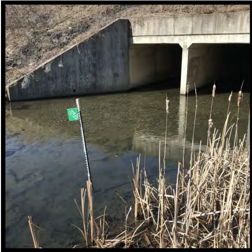
Trib 18788 Stream Gauge
